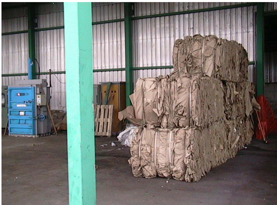
Specialized portable mechanical sorting equipment and baling storage area
