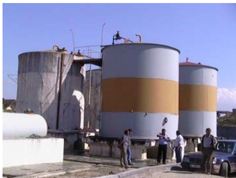
Oil treatment facility in Porto Romano
