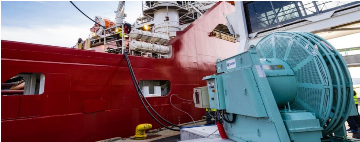
Figure 5.21 Onshore power supply to a ship at berth
