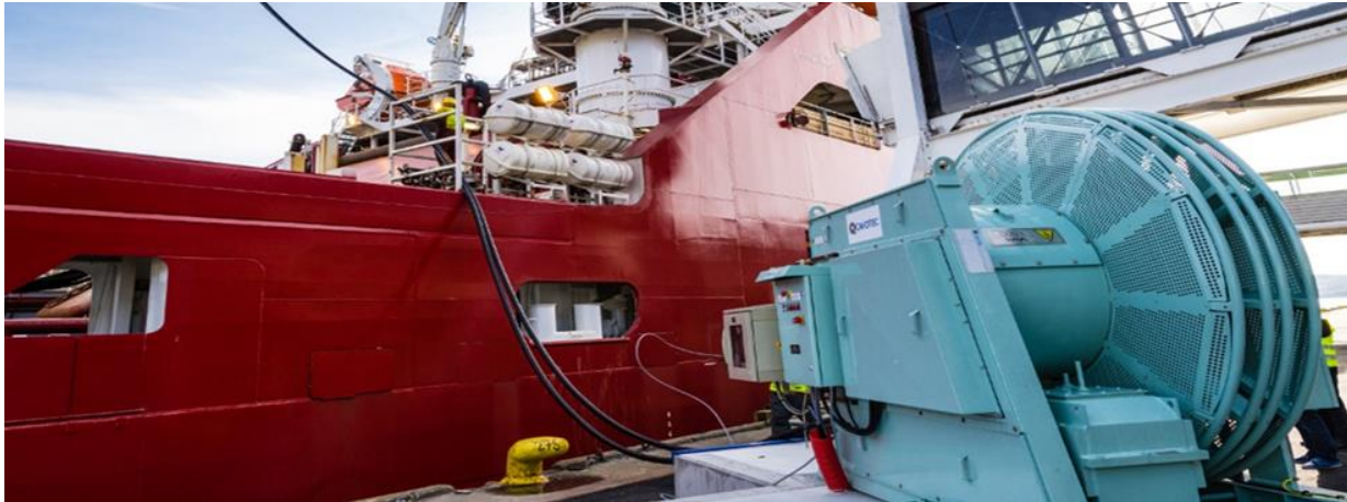
Figure 3.3 OPS to a ship at berth – Example no. 1
