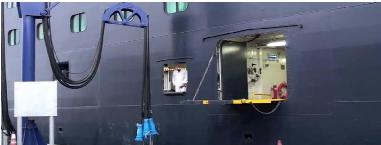
Figure 3.4 OPS to a ship at berth – Example no. 2
