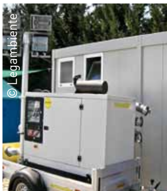
Electric generator in a tent city
